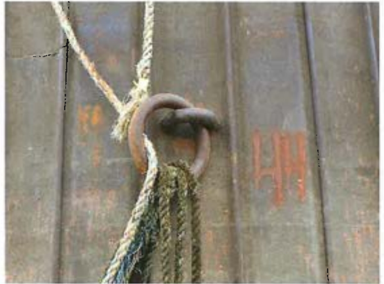
Photo 7: View of overstressed mooring ring on Sheet 45.
