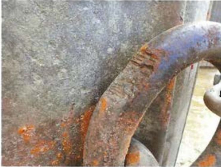
Photo 6: View of a missing section on the mooring ring.
