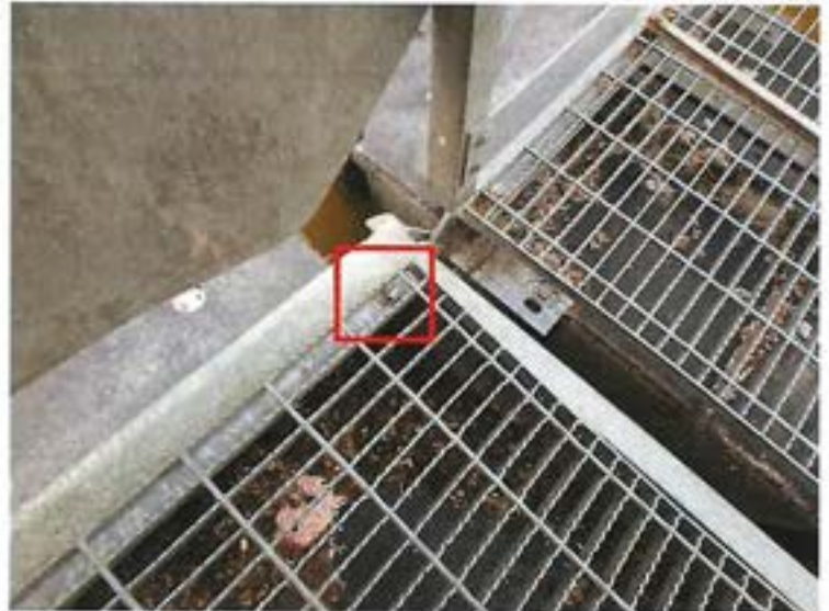
Photo 5: View of the missing grating clip on section 1.
