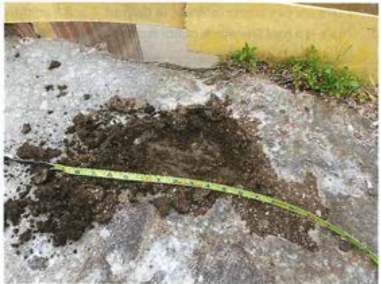
Photo 3: View of the spall in the cell cap.
