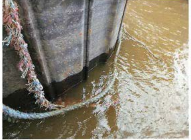
Photo 3: View of typical sheet pile condition at the waterline.
