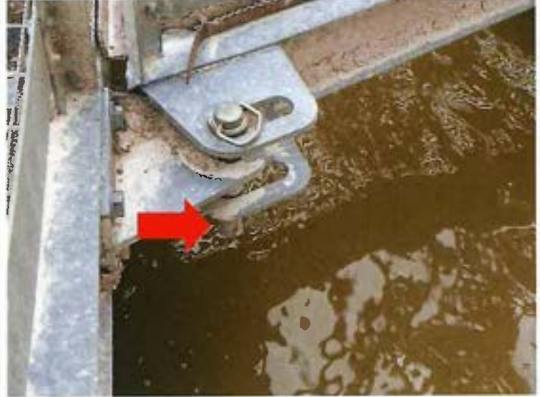
Photo 7: View of the missing lynch pin.
