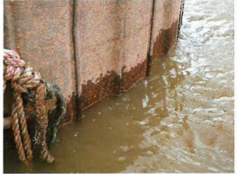
Photo 3: View of the typical sheet pile condition at the waterline.
