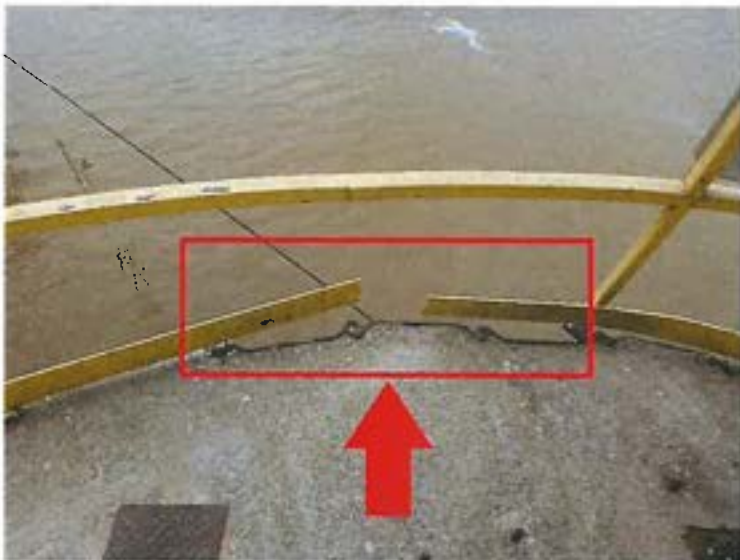
Photo 8: View of a broken toe kick over Sheet 41.
