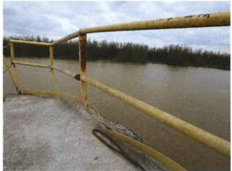
Photo 7: View of the impacted handrail.
