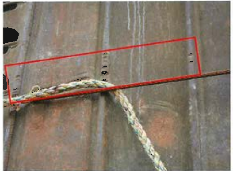
Photo 5: Sheets 46 to 1, abrasion damage from haul line
