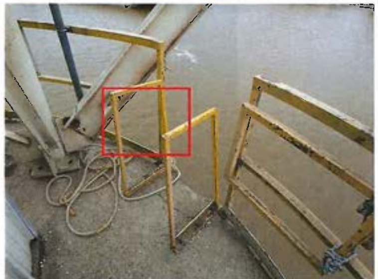
Photo 9: View of the missing safety chain over Sheet 1.
