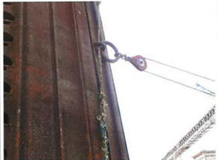
Photo 5: View of the haul line attached to the mooring ring at elevation 310 feet NGVD29.
