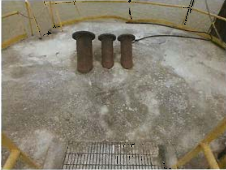
Photo 2: View of the concrete cell cap. Note the abandoned steel lines running into the cell cap.
