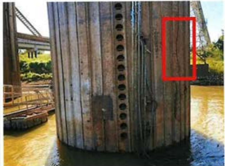
Photo 10: View of the impact damage on Sheets 43 and 44 (2021).
