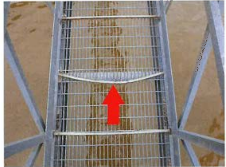
Photo 9: View of a typical bent traction bar.
