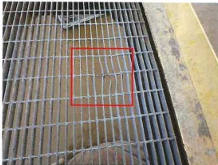
Photo 13: View of the broken grating on the walkway.
