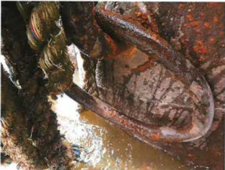
Photo 3: View of the overstressed mooring ring at El. 296 feet.
