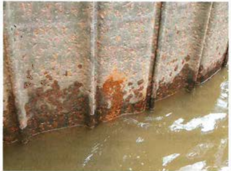
Photo 4: View of the typical sheet pile condition at the waterline.
